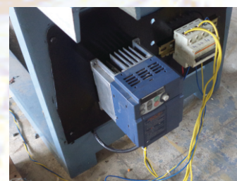
Electronic Drive Automation
